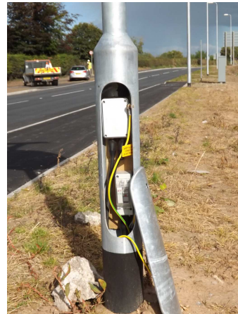
CEP4 Above Ground Solution
