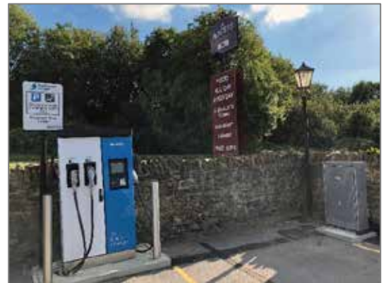
EV Distribution Pillar for Highways England supporting standard and rapid charging.
