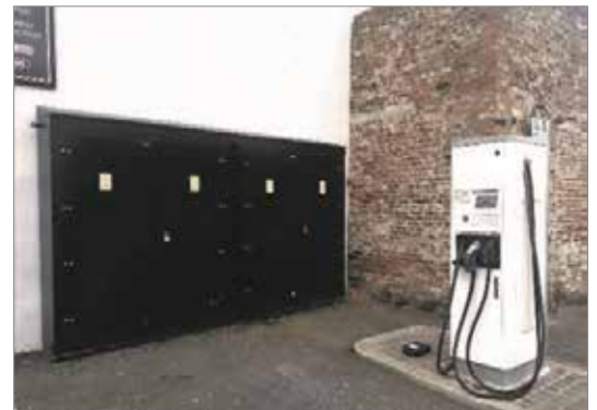
The brief for this project was for the pillar to be as streamline as possible to fit into the limited space available, but still have the capacity to contain all the required connections.
