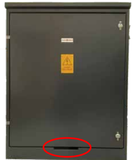
Cable Exit Tray
