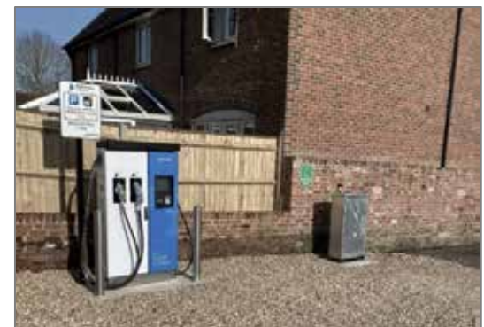
Another design for Highways England, this pillar provides all the power distribution needed for the charge point.
