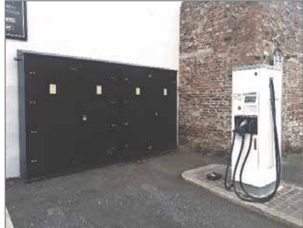
Bespoke, slimline pillar supplying EV Charges.
