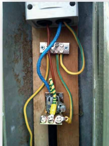
Example of CET 003 being used with EB42 earth block feeding Isolator with plastic gland plate
