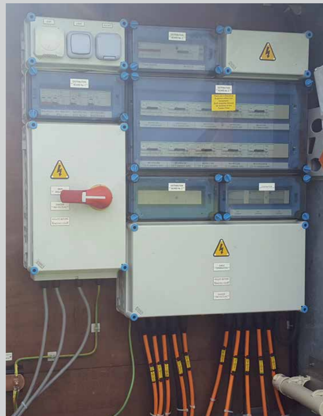
This is an example showing IP65 Distribution Panels for group switched lighting with electronic Passive Safety Disconnection.
